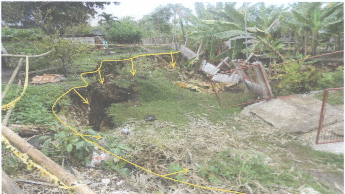
Cave roof collapse in Tagbilaran City, Bohol due to October 2013 Bohol earthquake
