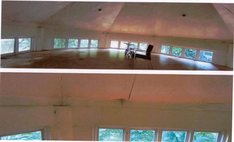
Dilapidated ceilings in the mezzanine floor
