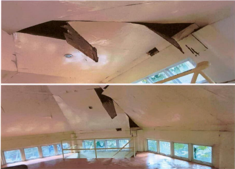
Dilapidated ceilings in the mezzanine floor
