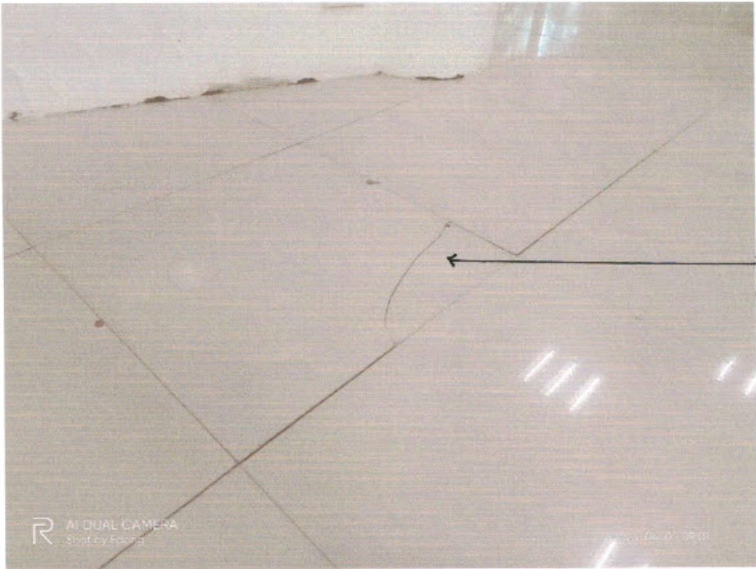
Existing floor tiles (sira-sira na talaga)
